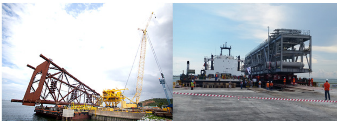
Chevron Project Offshore Platforms
